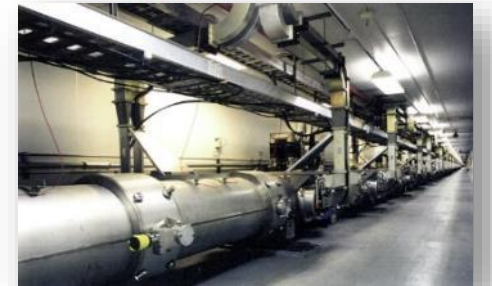
Cryomodules in the accelerator tunnel
