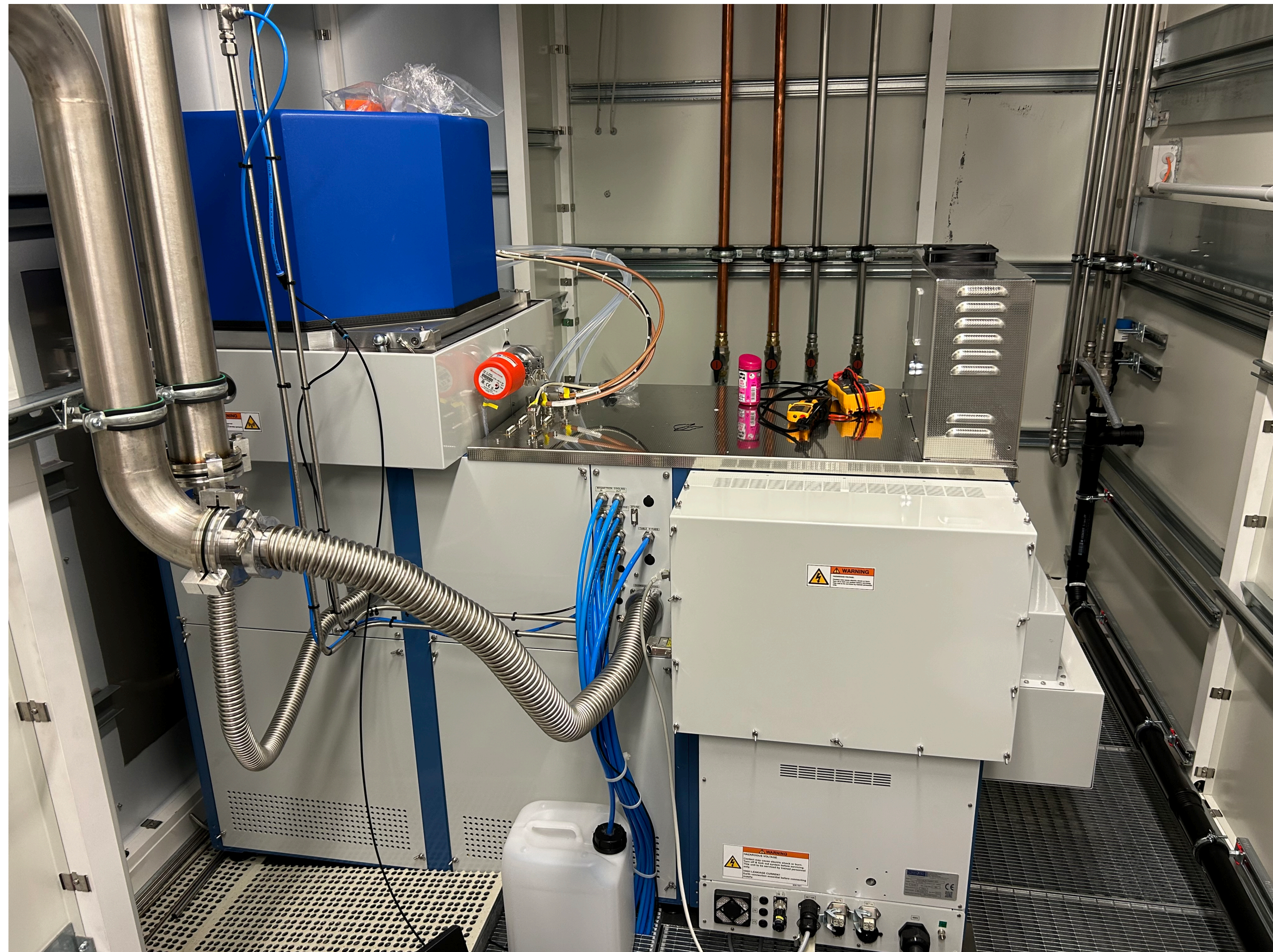
Rest of machine in technical corridor
