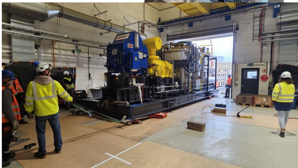
Compressor skid arrived last week
