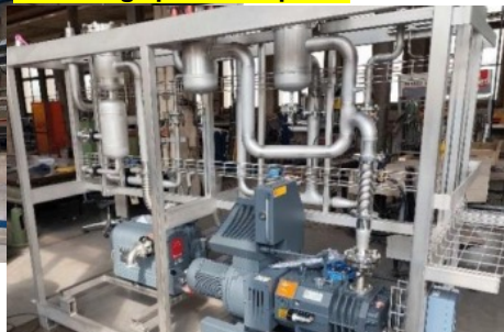
WCS Purge panel completed
